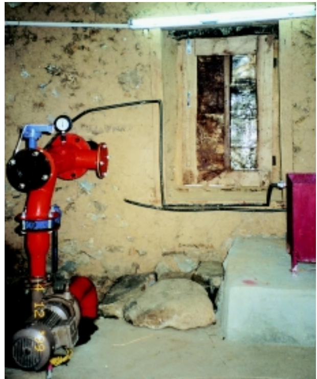
Pump as Turbine installed in Gotikhel VDC, Lalitpur
