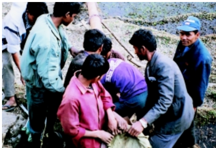
Community members engaged in the installation of penstock pipe in Duni VDC, Achham
