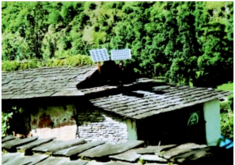
Solar Home System installed in Pokha Phant, Myagdi
